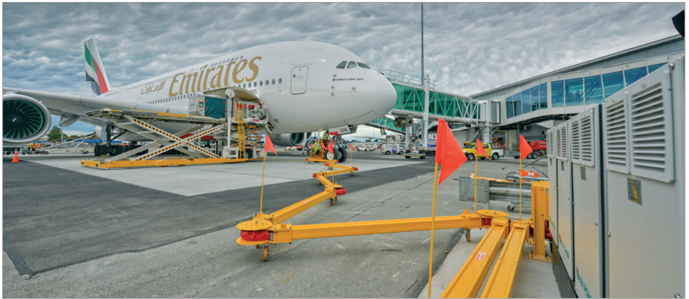
Figure 10: Fixed Ground Power Unit for an A380
